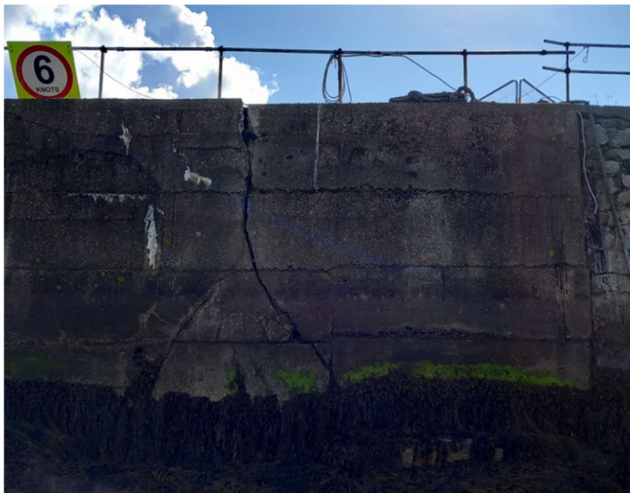
E: Structural Failure to the West of the Central Causeway, looking east
